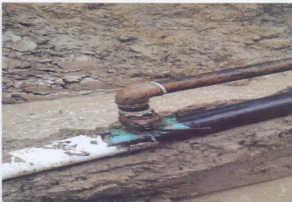
Exposed pipe showing course of spill.
